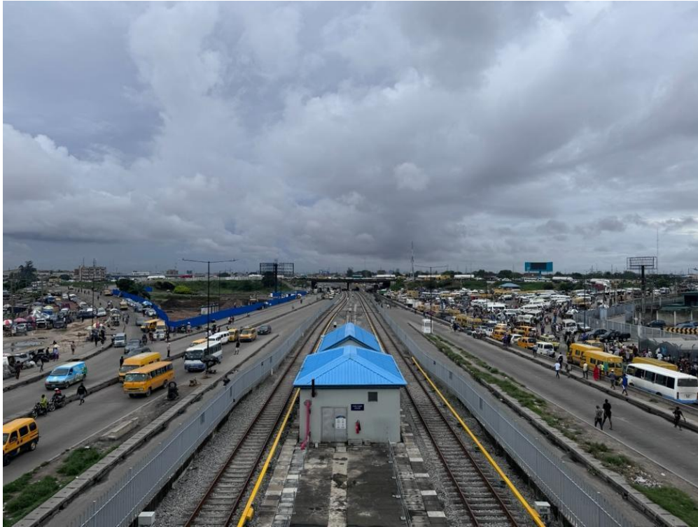
Figure 12. A power generation room for the Blue Line as seen from the pedestrian footbridge adjoining Mile 2 station. Photo credit: Temilade Sesan.
